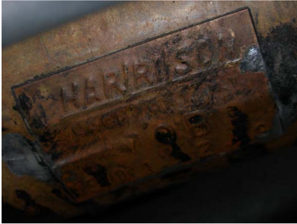
Expansion Tank – Harrison Industries, Lockport, NY. Code 70B – 1970 February
